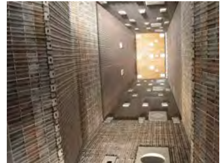
Looking up inside the new, 35-meter high waste incineration boiler at Spittelau in Vienna.
