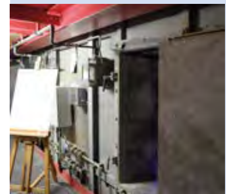
One unusual aspect: The project presentation and press conference were held inside the new boiler (the "front door" of which can be seen here).
